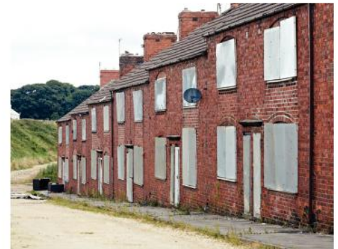
▲ Derelict housing in a run-down area in Doncaster. The council will replace it all.
